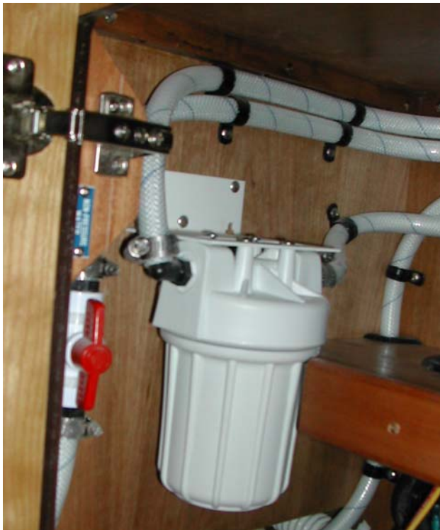
“Shurflo” RV-5UC water filter below galley.
