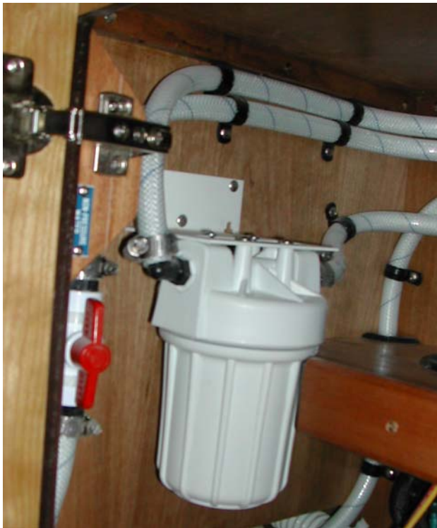
“Shurflo” RV-5UC water filter below galley.
